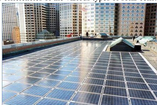
Fig. 3. Boston, Massachusetts' Williams Building. A total of 372 modules were used, giving the system a 31-kW output.
